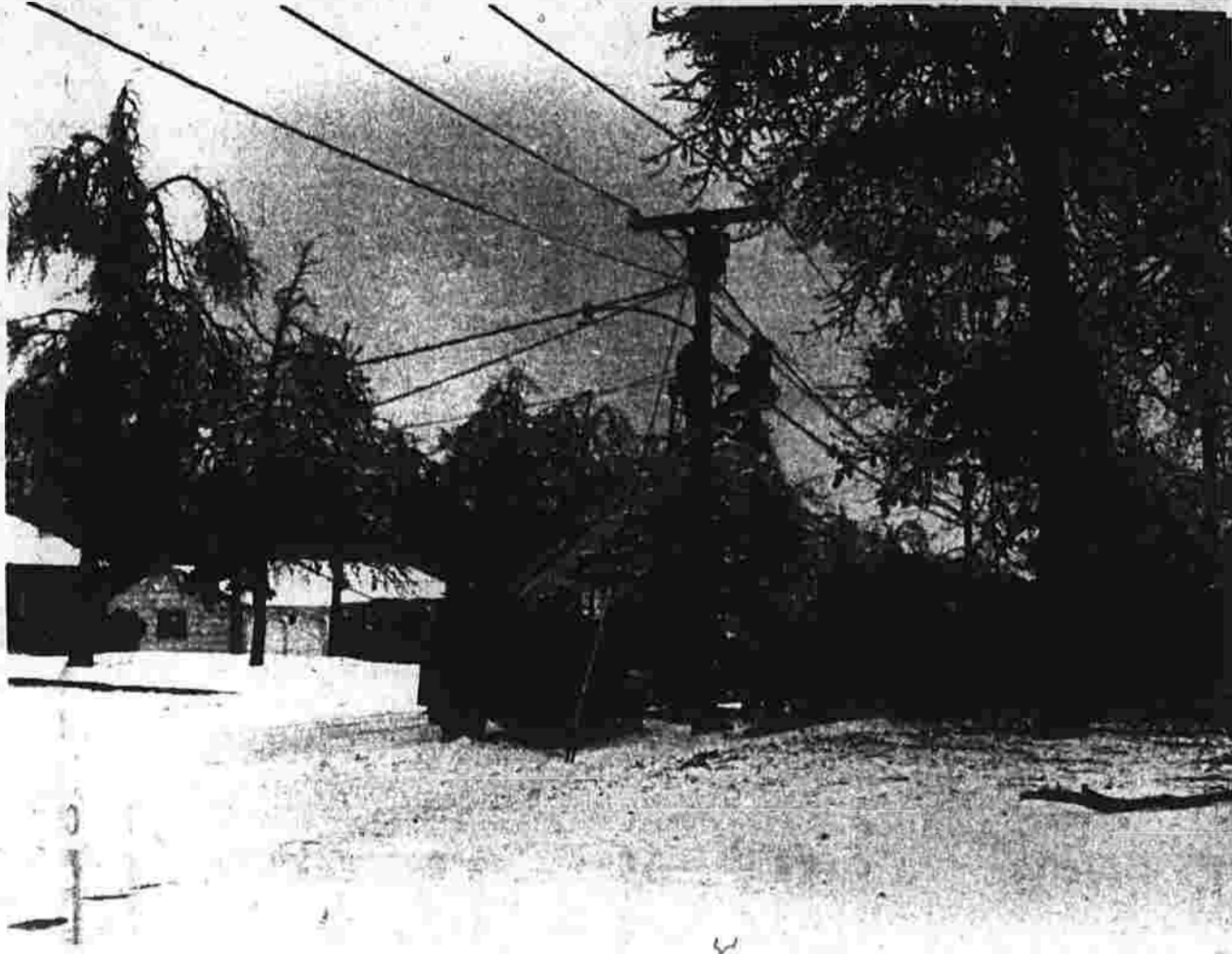
With literally hundreds of downed power and telephoto lines, utility crews from throughout the state and out of state have been brought in to restore service in Manchester and surrounding communities. Main truck line service has top priority with individual service connections next in line. (Herald photo by O'Hara)
